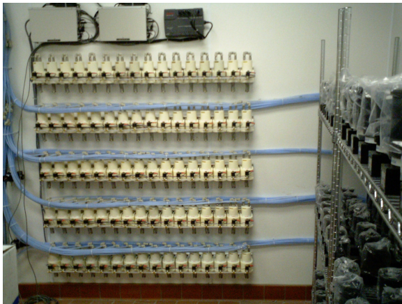
The above picture shows five sixteen-pump rails mounted near the bottle reserve.
